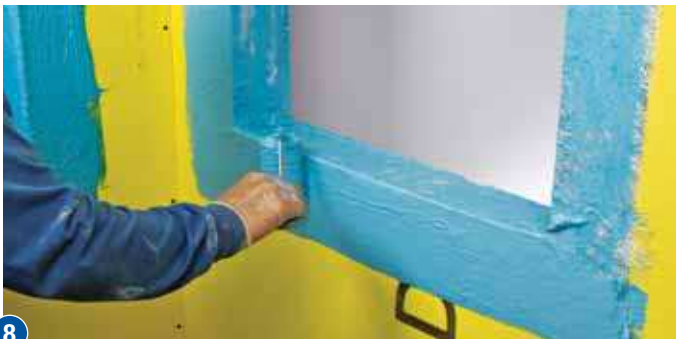
8 Apply second coat of 30 wet mils of fluid applied membrane to encapsulate LiquiFiber. Apply same day as LiquiFiber.
