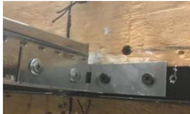
FIGURE 18 – CERTAINTED LBRC ANGLE CLIP (WITH TWO SCREW ATTACHMENT AT EACH LEG) FIXED WALL ASSEMBLY WITH WALL ANGLE (WA14-14) IN SECTIONS 4.2.6, 4.2.9, 4.2.10, 4.2.11 AND 4.2.12
