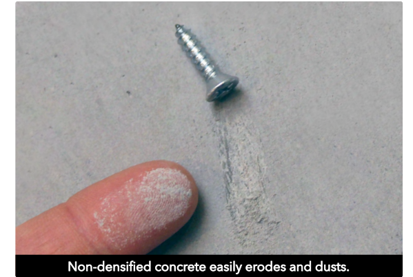
Non-densified concrete easily erodes and dusts.
