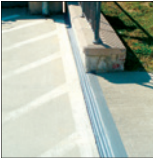
DSM System technology provides a structural joint sealant solution. Here DSM is installed at the top of a ramp where a driveway transitions from on-grade to supported slab and from deck-to-deck to deck-to-wall.
