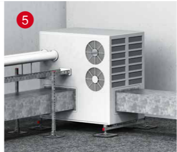
5 Air handling units
