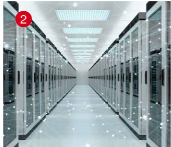
2 Hot / Cold aisle containment
