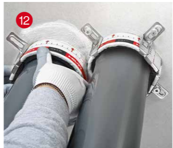
12 Piping and ventilation
