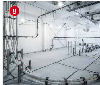
8 High-voltage cabling supports
