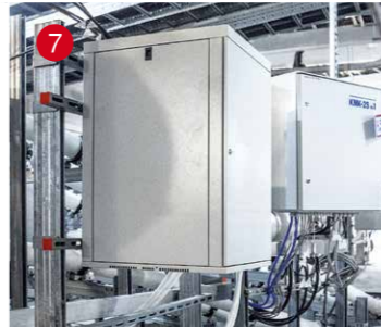
7 Equipment supports and platforms
