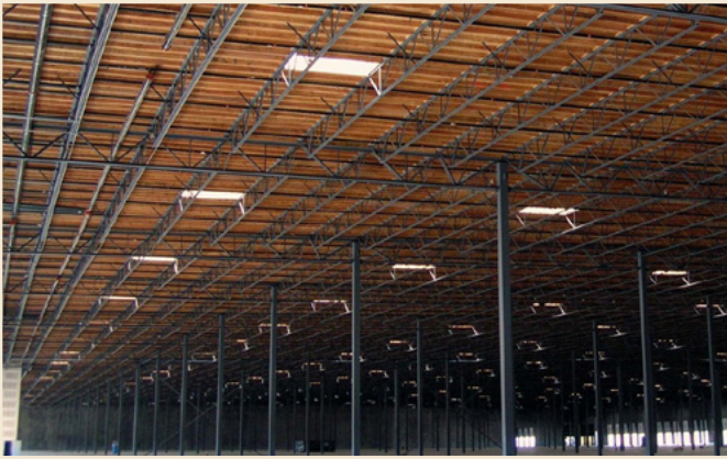
Type I: 1.2 million SF panelized roof system used PyroGuard™ lumber and plywood. Phoenix, AZ.
