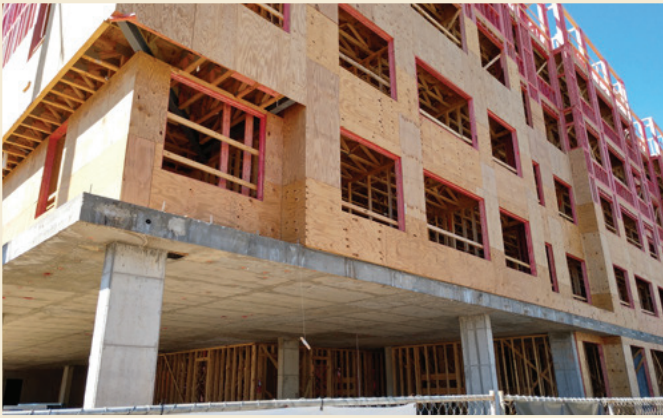
Type III with Type I podium: PyroGuard™ used both above and below the podium. Charleston, SC.
