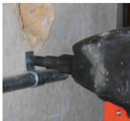
12HSMP034 clip assembly used to secure conduit
