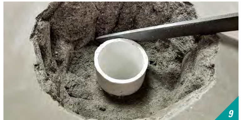
Using a file, debur the pipe and clean out all of the remaining debris around and inside waste pipe.
