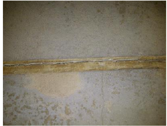
Photo #10 - cohesive failure
