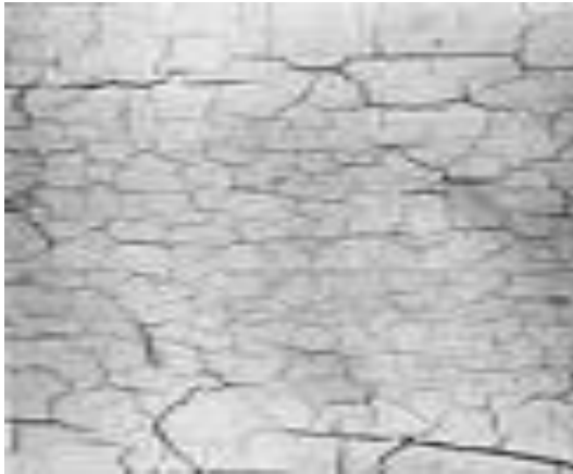
Photo #9 - Sealant aging w/ cracks
