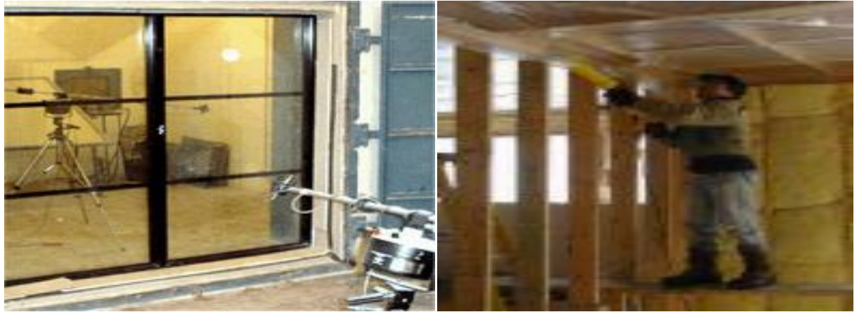
Picture #5: Sealants should be designed to maintain the STC rating of the existing wall by sealing penetrations.
