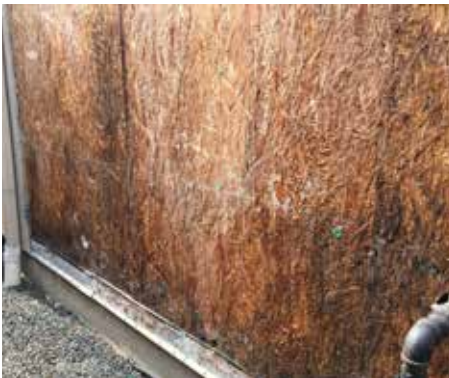
Image 2: Saturated oriented strand board (OSB) sheathing due to insufficient drainage and insufficient vapor control behind stucco on a 3-story townhouse in a hot-humid climate, 8 years after construction. The stucco cladding was installed over two layers of mechanically-fastened building wrap. While this wall assembly complies with the current building code and the windows and penetrations were flashed correctly, two layers of building wrap do not provide enough of an air space behind the stucco to (1) relieve hydrostatic pressure, (2) act as a capillary break and receptor for capillary water and (3) facilitate hydric redistribution and moisture removal by air change.
