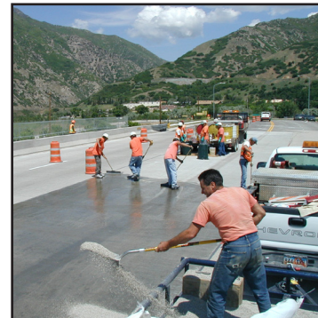
When material levels, broadcast aggregate slowly, allowing it to settle into epoxy.
