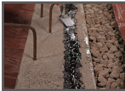
Onto Interior Grade Beams at Impediments: Seal Drago Wrap to concrete with Drago Mastic.
