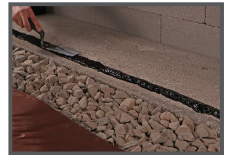
At a Location Designated by the Design Team: Seal Drago Wrap to concrete with Drago Mastic .
