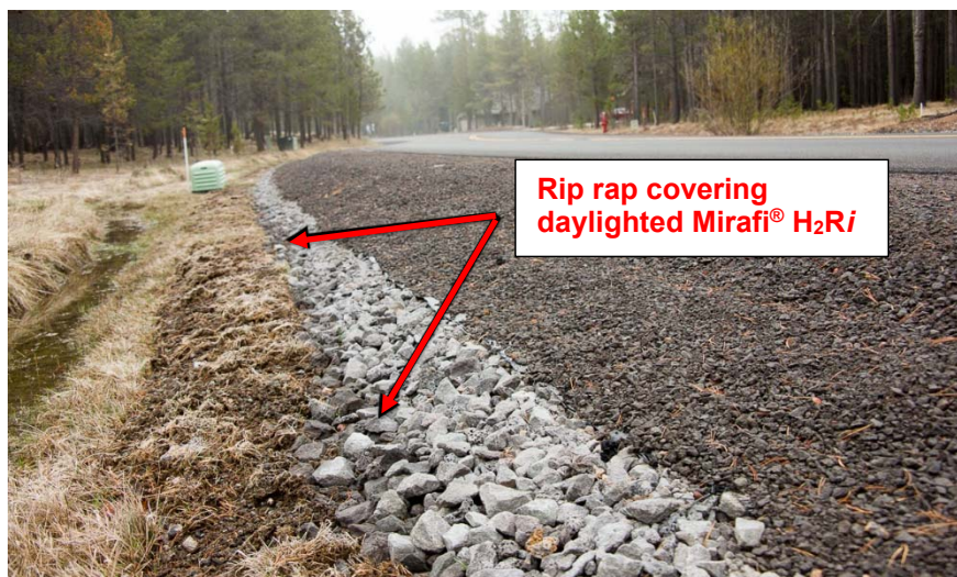
Image 9 - Daylighted Installation Using Rip Rap to Cover the Exposed Edge of Mirafi ® H 2 Ri.
