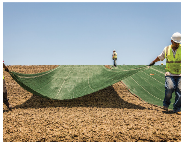
Figure 4(b): Project photo of PROPEX Pyramat 75 being placed on the slope face
