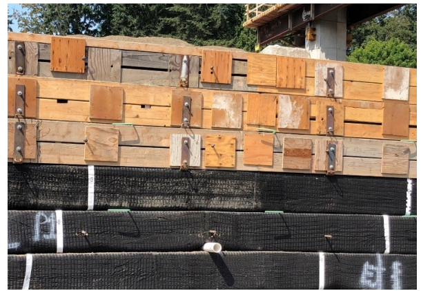
Figure 11(b): Project photo of MIRAGRID XT geogrid wrapped face MSE wall under construction
