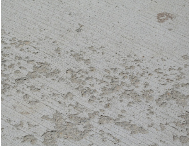
New Concrete Exposed to the Damaging Effects of Mild Freezing at an Early Age
