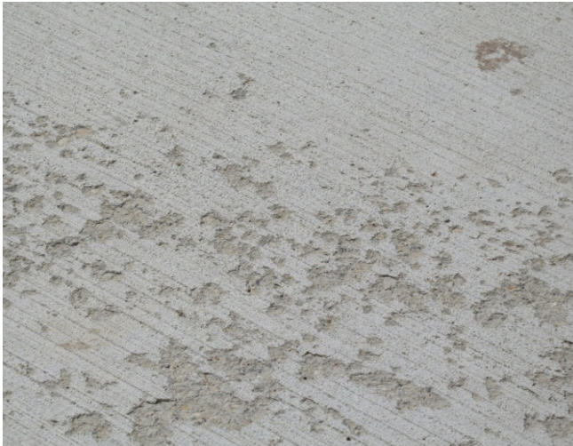
New Concrete Exposed to the Damaging Effects of Mild Freezing at an Early Age
