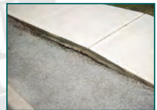
Ignoring expansion joints in pavement construction can lead to various problems.
