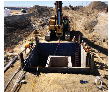
South Lathrop Commons, California, USA Wet Well/Pump Station • Xypex Bio-San C500, Xypex Megamix II with Bio-San
