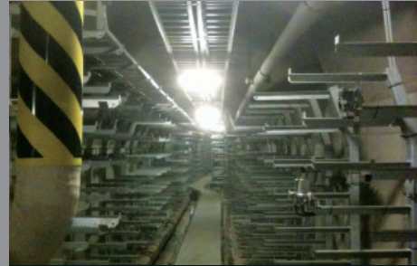
Prague City Utility Tunnels, Czech Republic
